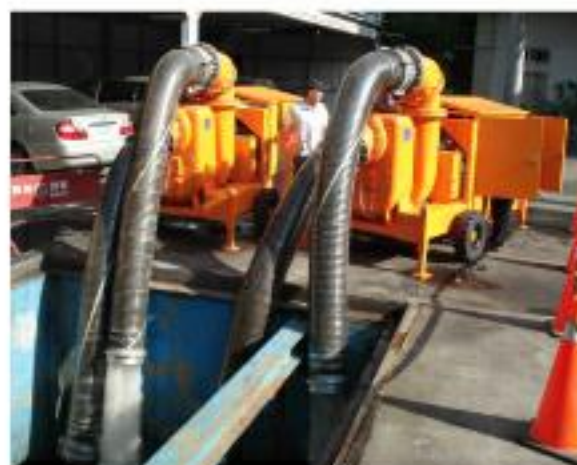
Pump Continuous Running Test
