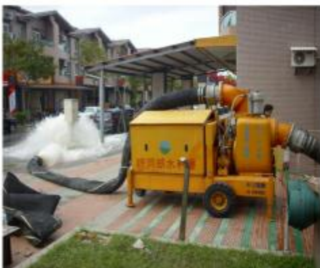
Draining water at basement
