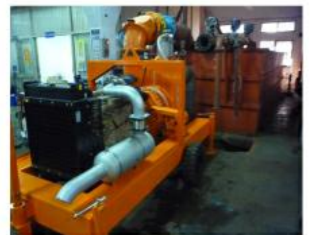
Pump Performance Test
